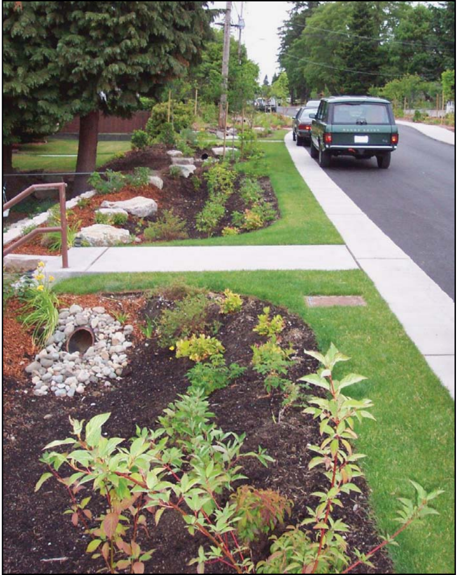
Seattle Public Utilities has retrofitted several blocks of city streets with LID features. Stormwater runoff is directed from narrow, curbless streets to planted bioretention swales for treatment and infiltration. Seattle found that the new design costs less than conventional construction that provides comparable water quality treatment. / Seattle Public Utilities
