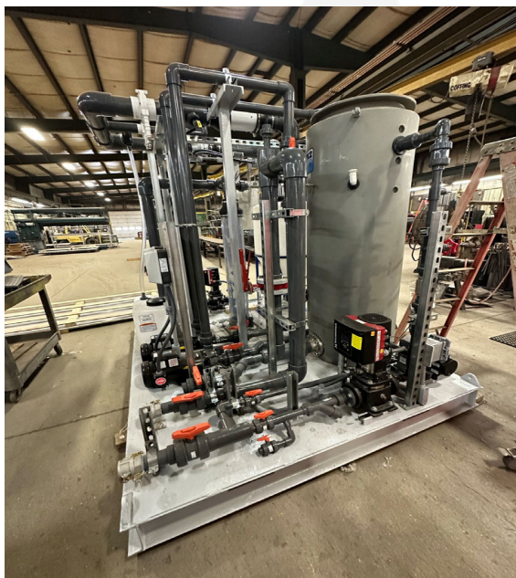
8' x 6' Skid-mounted pilot scale 2-6 gpm
