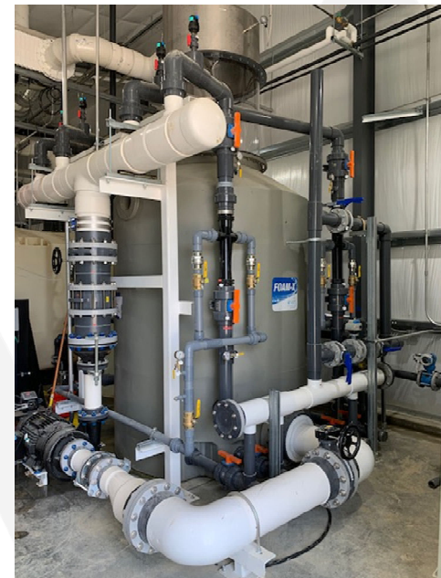
14' High Permanent Install 50 to 150 gpm
